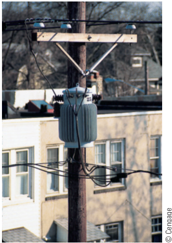
Figure 32.18 The transformer on this power pole steps down AC voltage from 4 000 V to 240 V for distribution to individual residences.
